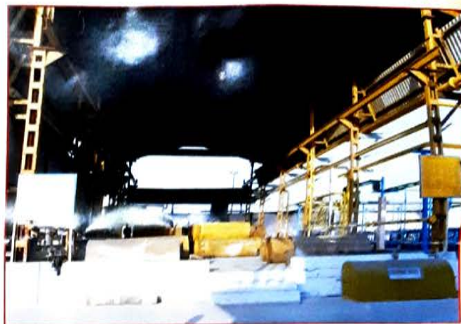
Chlorine handling shed at CETP, Nandesari
