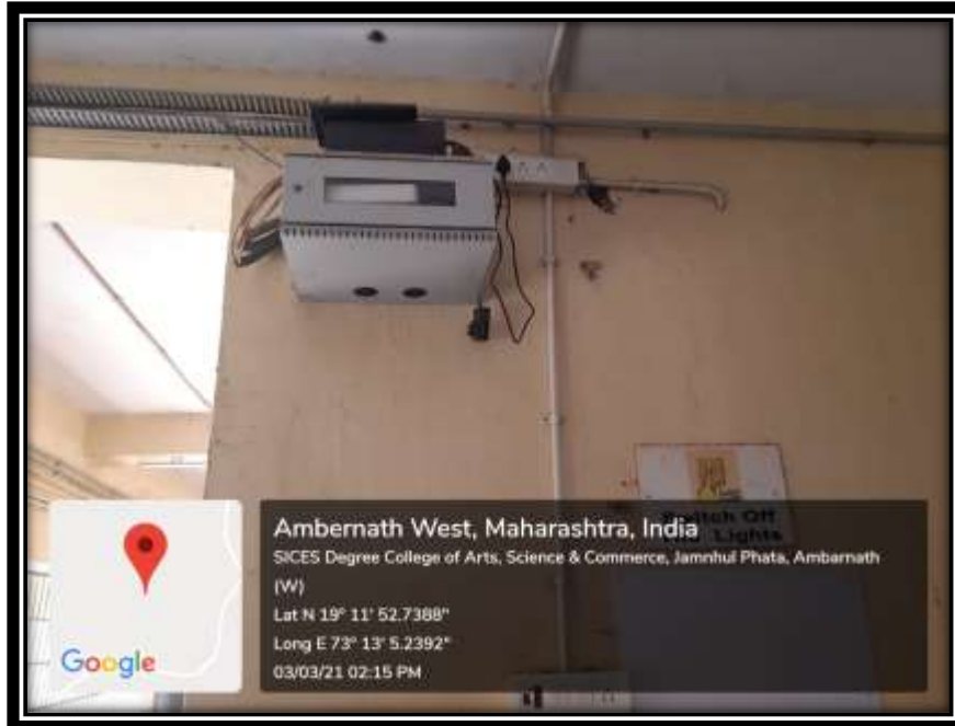
Internet Server 2 nd Floor
