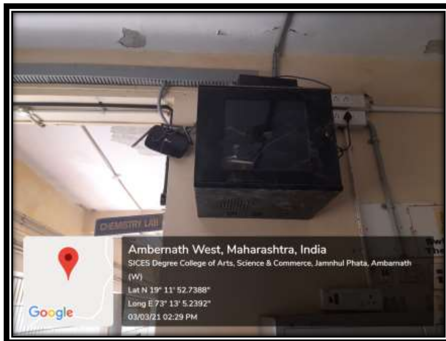
Internet Server 3 rd Floor Internet Facility
