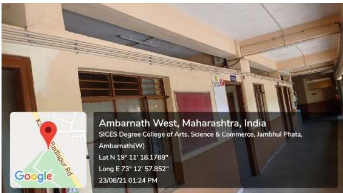
II Floor walls showing cables for CCTV and Speaker of Central Mic system
