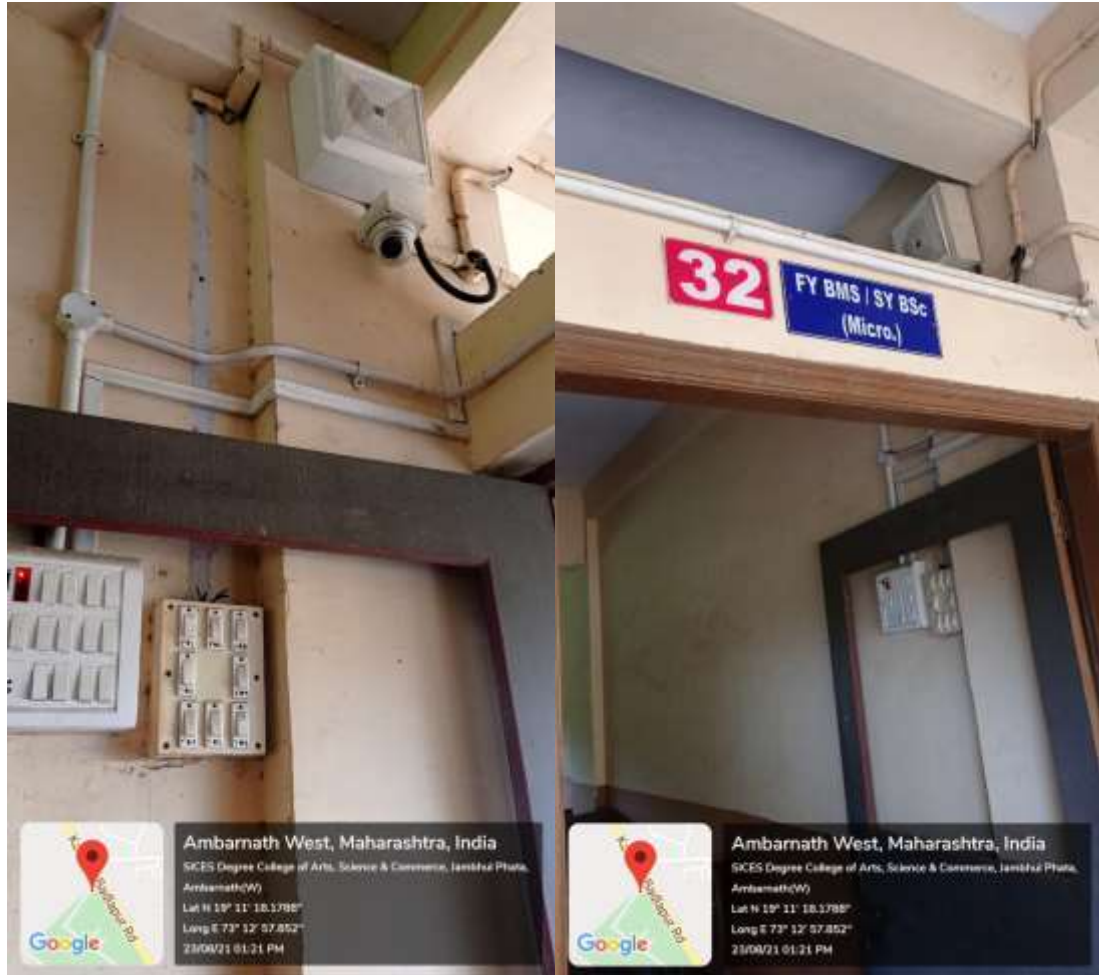
CCTV and Speaker in Class room
