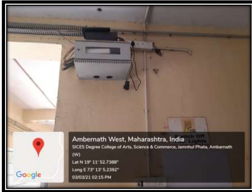
Internet Server 2 nd Floor
