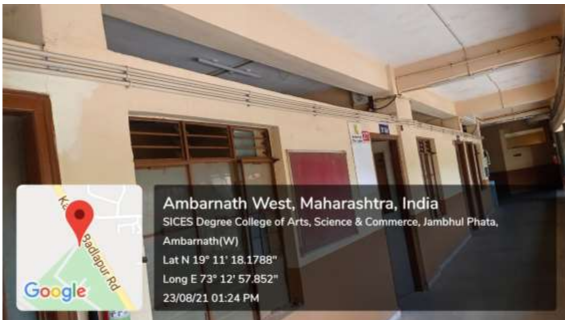
II Floor walls showing cables for CCTV and Speaker of Central Mic system
