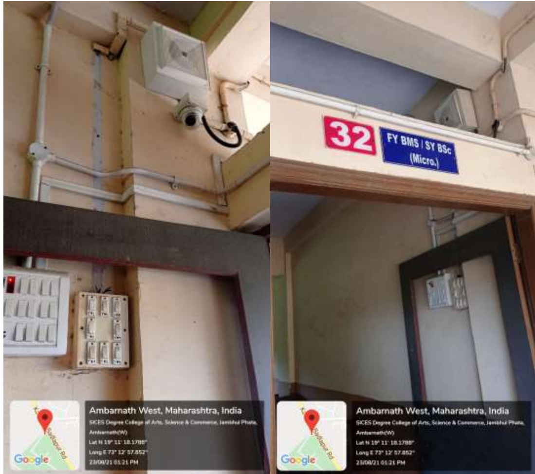
CCTV and Speaker in Class room
