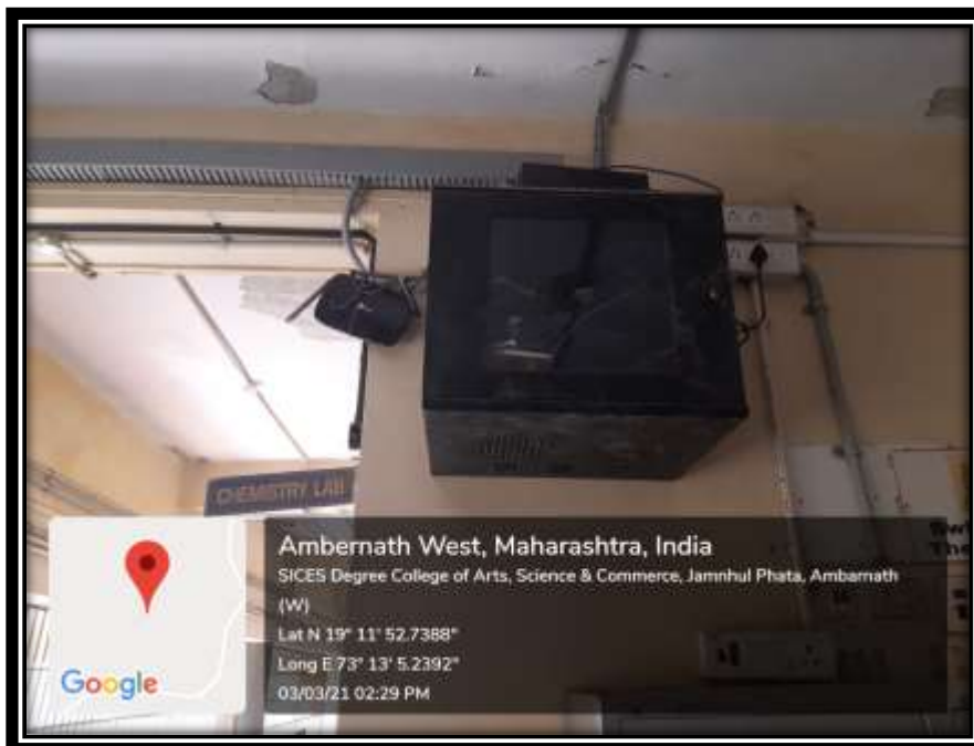
Internet Server 3 rd Floor Internet Facility
