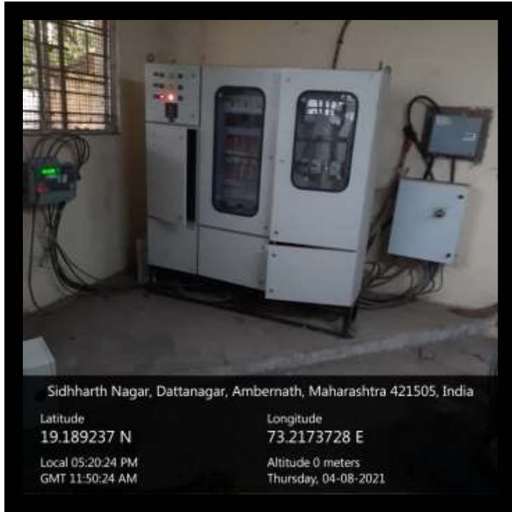
Electric panel room
