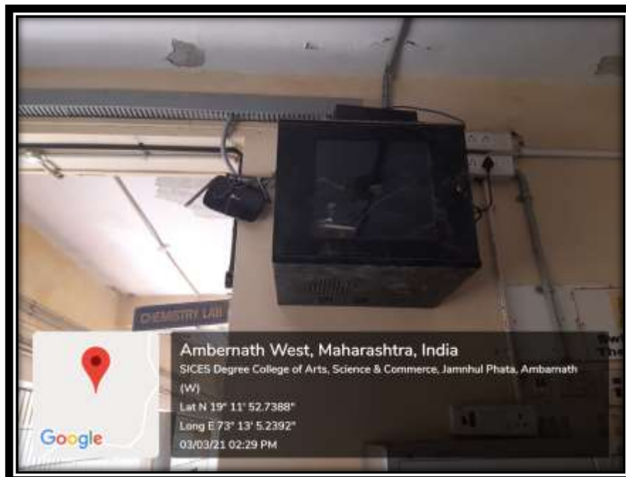
Internet Server 3 rd Floor Internet Facility
